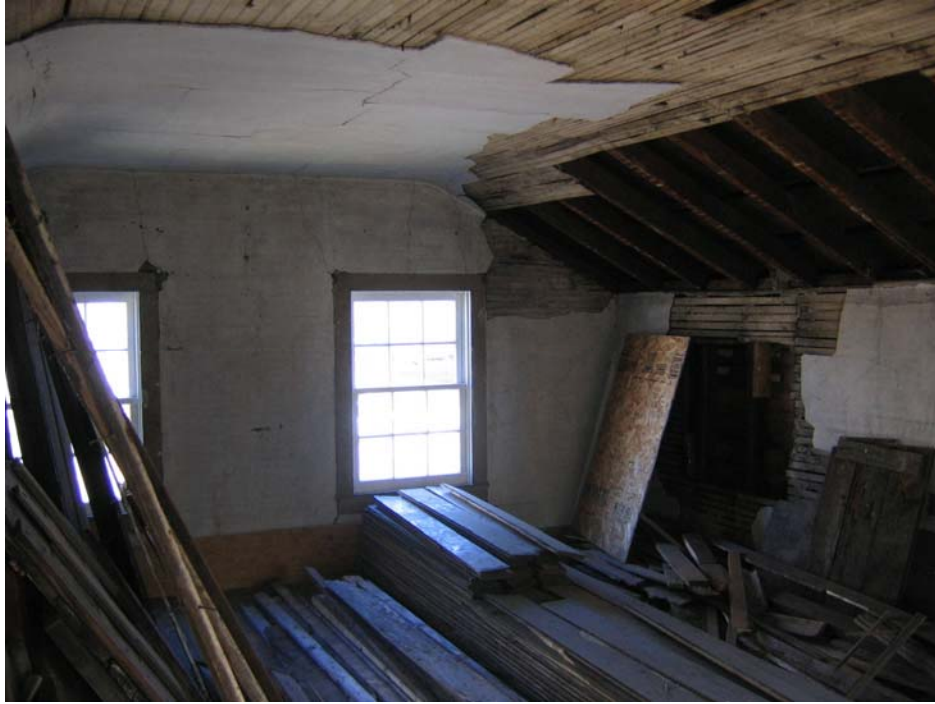
A view of the second floor looking north. Note the large pieces of lath and plaster missing.
