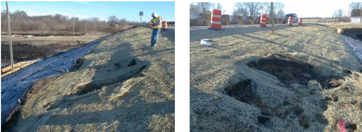
Figure 2.4: Pictures of surficial slope failure along CTH A near Burlington, Wisconsin (embankment slope).
