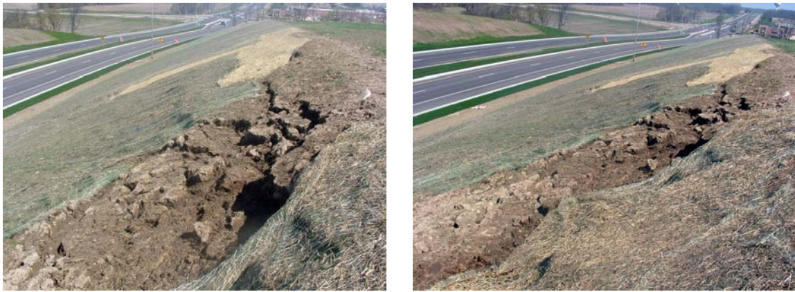
Figure 2.3: Pictures of surficial slope failure along STH-164 in Waukesha County, Wisconsin (cut slope).
