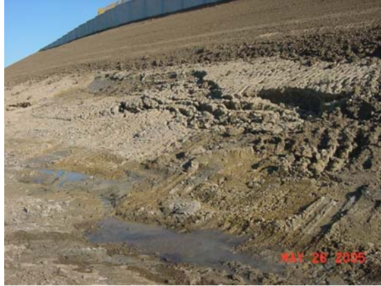
Figure 2.28: Shallow slope failure at STH-16 with water seeping out of the slope face.
