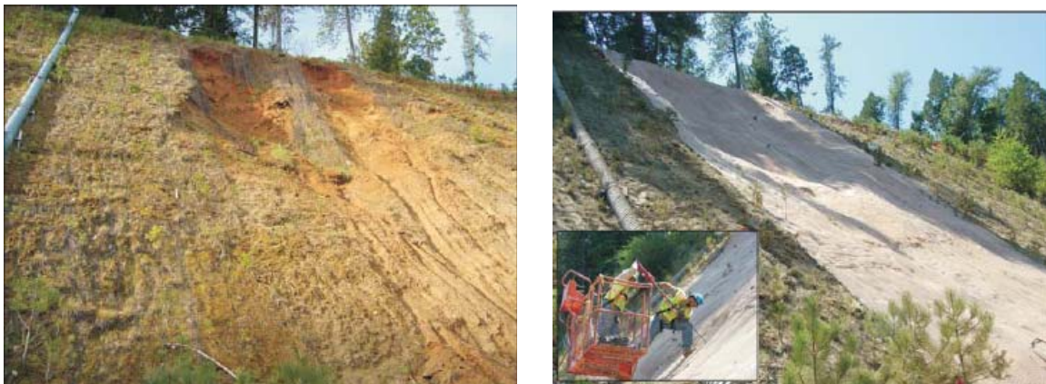
(a) Surficial slope failure
