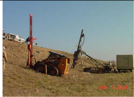
(d) Ingersoll Rand ECM350 pneumatic hammer drill (background) and drop-weight hammer rig (foreground)
